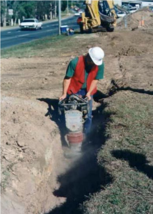
Initial backfill compaction being undertaken with a hand held compactor - a controlled operation.
