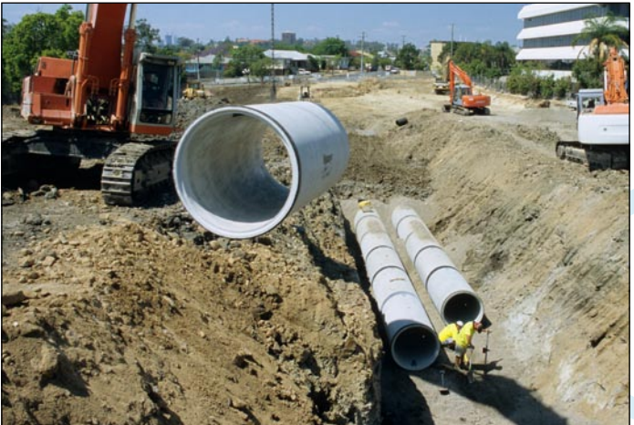
Example of a good installation - trenches are neatly excavated and the pipes are progressively backfilled.
